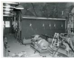
AEC Air Handling Equipment (25 June 1957) (1983.63.111)
