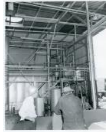
Inside new boiler house AEC Compound (26 Sep 1956) (1983.63.115)
