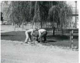
AEC Fire Hydrant (Oct 1957) (1983.63.127)
