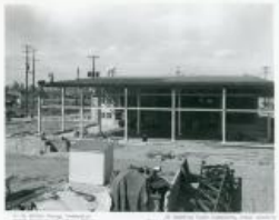
Starting construction SS Sampling plant expansion south dock showing new concrete slab (4 Sep 1956) (1983.63.145)
