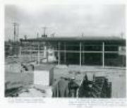
Starting construction SS Sampling plant expansion south dock showing new concrete slab (4 Sep 1956) (1983.63.145)
