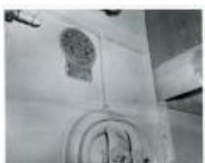
Grand Junction boiler House AEC Compound (1983.63.112)
