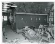
AEC Air Handling Equipment (25 June 1957) (1983.63.111)
