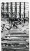
Photo and negative of culvert construction under Rock Creek trestle on the D&SLRR (1990.10.79)
