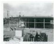
Starting construction SS Sampling plant expansion south dock showing new concrete slab (4 Sep 1956) (1983.63.145)
