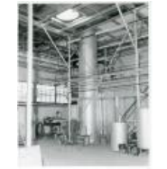
Grand Junction AEC Compound Boiler house inside (26 Sep 1956) (1983.63.116)
