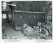
AEC Air Handling Equipment (25 June 1957) (1983.63.111)
